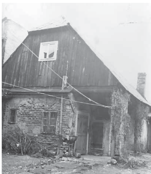
Fig. 3 Opatovina 21, house, western (courtyard) front (MK-UZKB-KOZ, photo by Lj. Krtelj, 1965, inv. ref. no. 9529)
